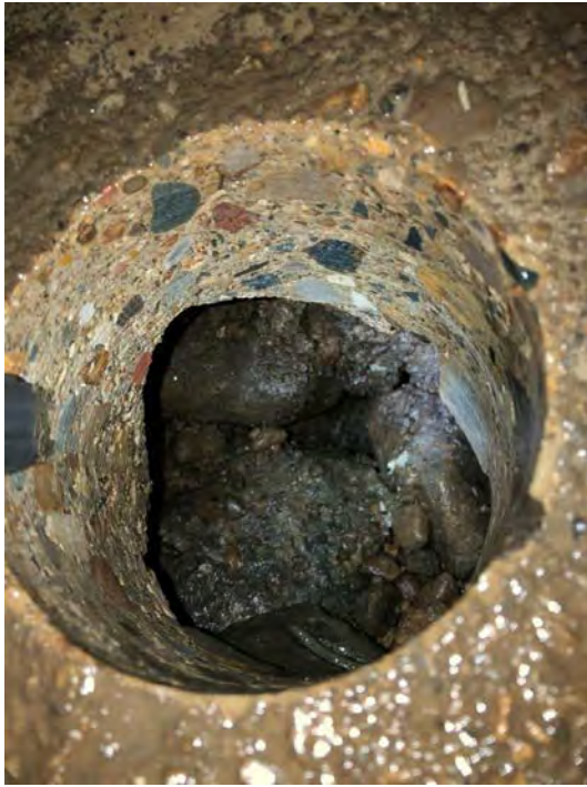
Photograph #1: Void Under Basement Slab
