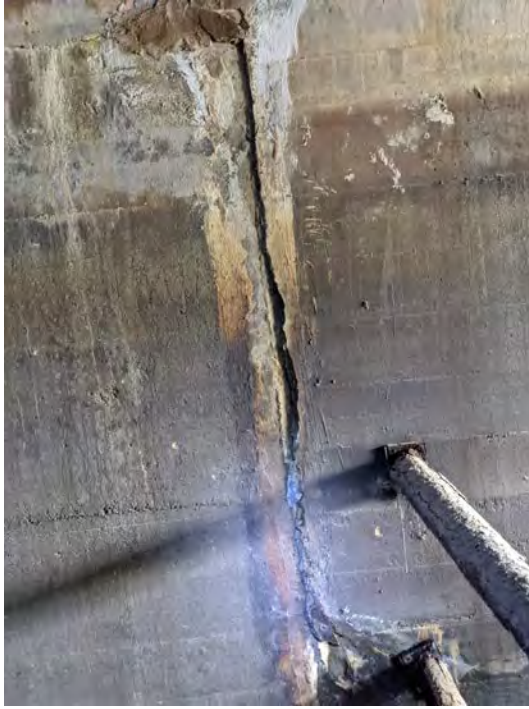
Photograph #7: Crack on South Wall of Headrace
