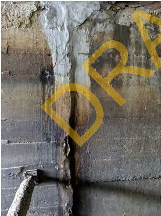
Photograph #8: Crack on North Wall
