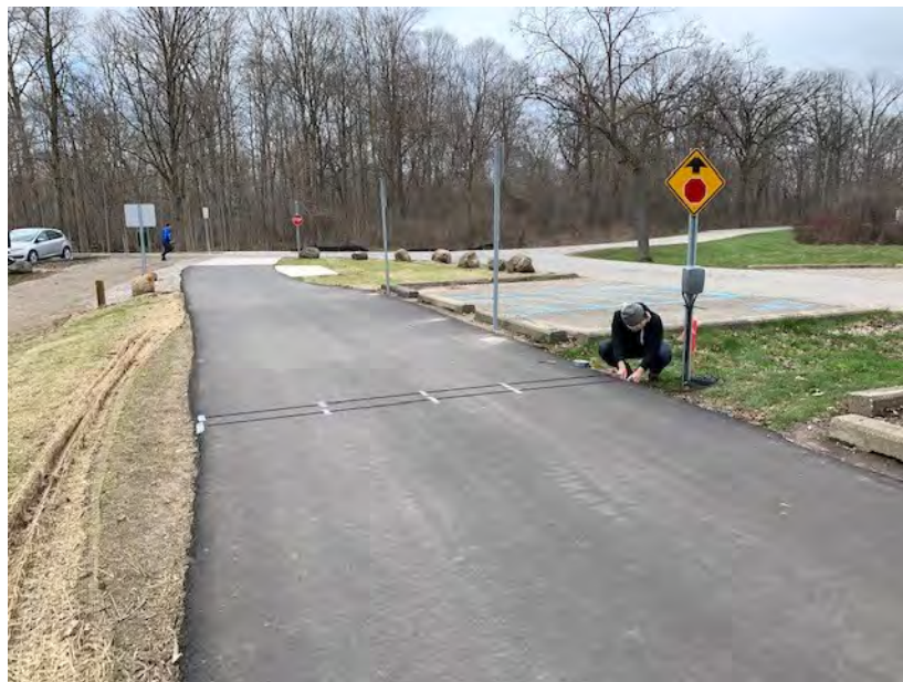
Border to Border Trail Eco-Counter installed at Dexter-Huron Metropark
