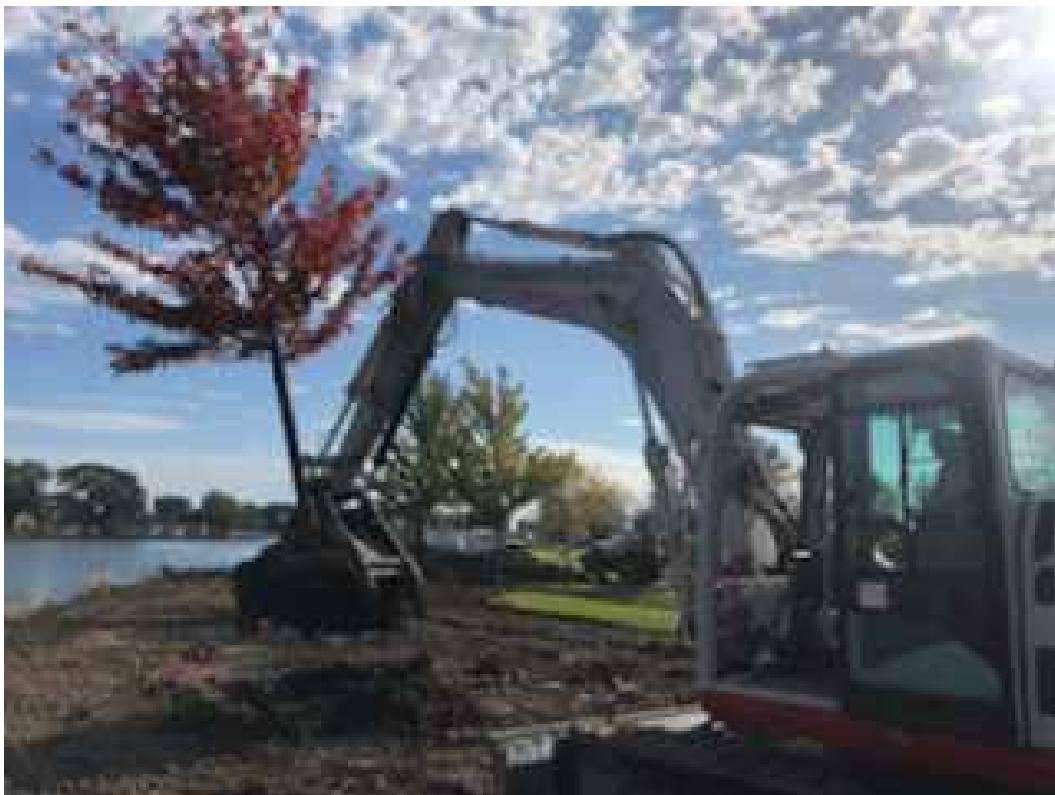
Figure 4: NRC prepares to relocate a young maple tree as part of the shoreline restoration project at Lake St. Clair Metropark.
