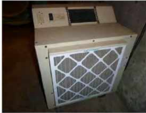
Image 81: Dehumidifier for Wave Pool Equipment Space
