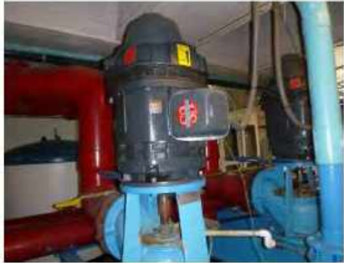
Image 55: Vertical Recirculation Pump
