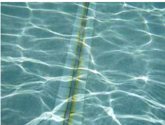
Expansion joint staining
