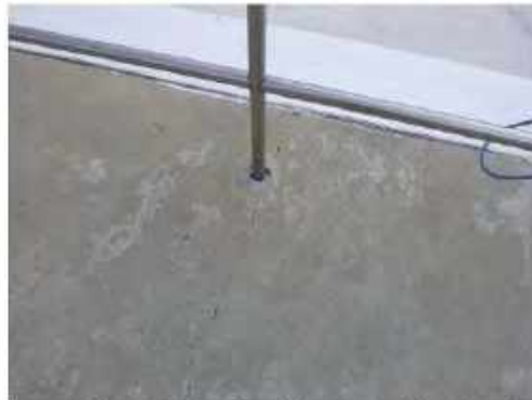
Image 36: Hairline Cracking at Railing Anchor
