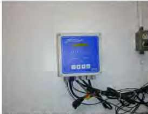
Image 75: Water Chemistry Controller
