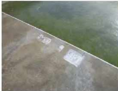
Image 28: Faded Painted Deck Markings
