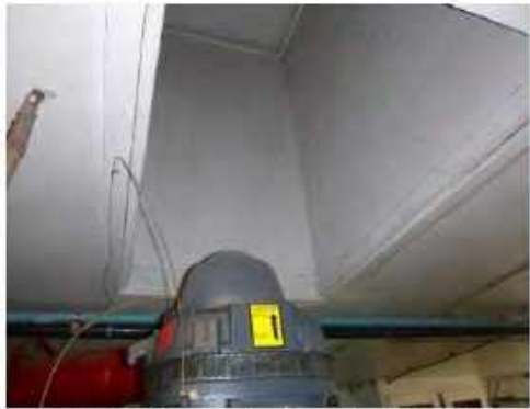
Image 57: Overhead Access for Servicing Recirculation Pumps
