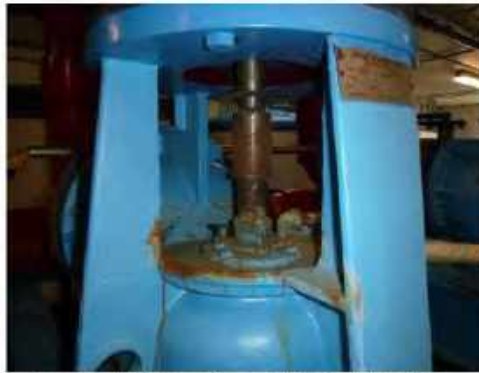
Image 58: Corrosion at Vertical In-Line Split Coupled Pump
