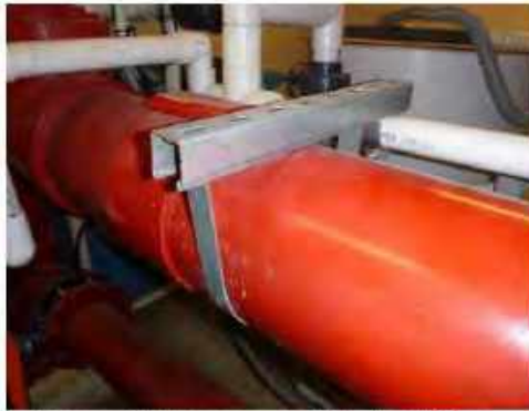
Image 47: Unsupported Strut and Pipe Guides / Straps
