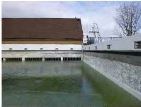
Image 9: Deteriorated Finish & Substrate along Side and End Walls
