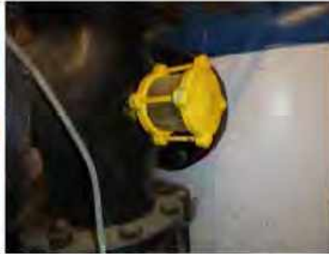
Image 54: Backwashing Sight Glass
