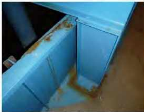
Image 63: Corrosion at Coated Steel Surge Tank
