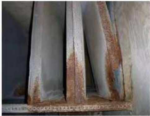
Image 82: Corroded Baffles in Equipment Room
