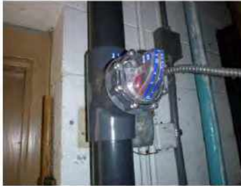
Image 45: Sprayground Flo-Vis Flow Meter
