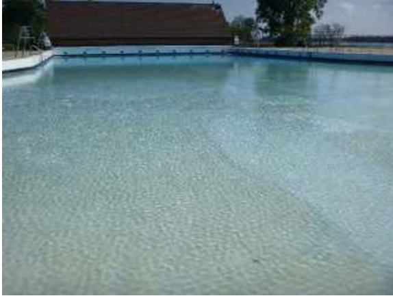
Visible repairs to the pool surface
