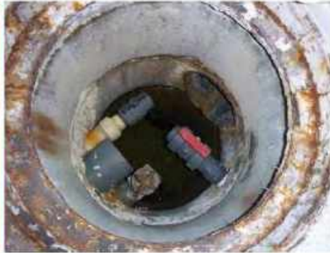
Image 40: Waste Pit Valves
