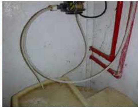
Image 74: Acid Feed Pump and Poly Piping
