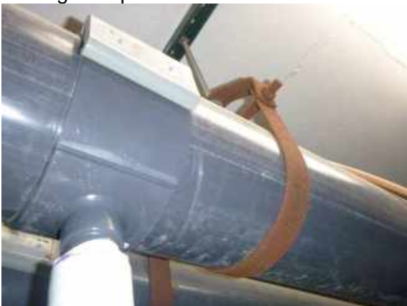
Corroded pipe hanger
