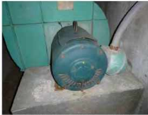
Image 83: Motor and Unsupported Fan
