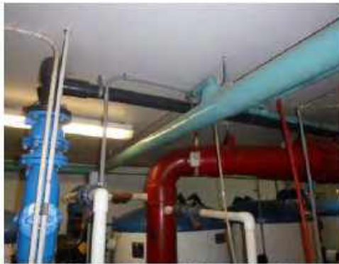
Image 73: Chlorinator Side Stream Taps
