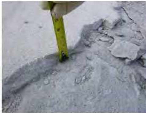
Image 3: Delaminated Plaster Finish
