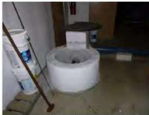
Image 52: Sanitary Waste Pit
