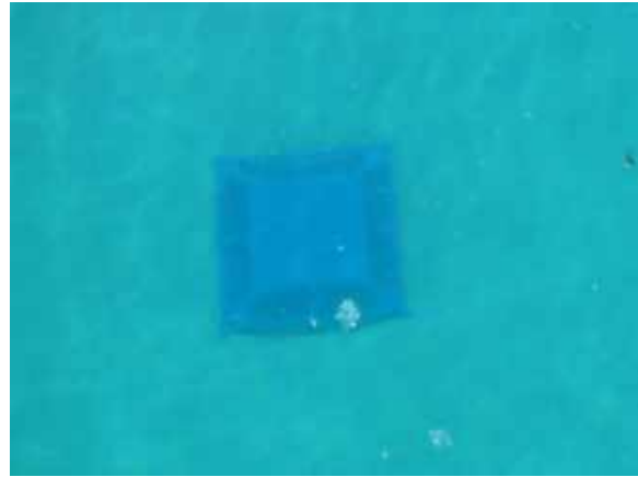
Pool drain not flush to pool surface
