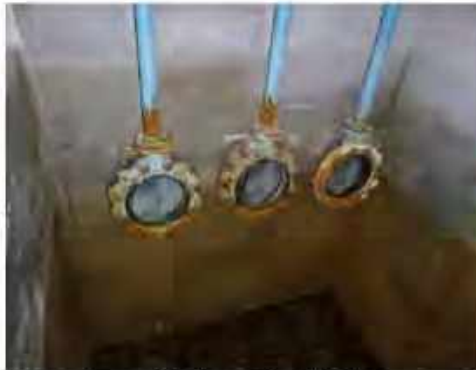
Image 37: Surge Tank Valves
