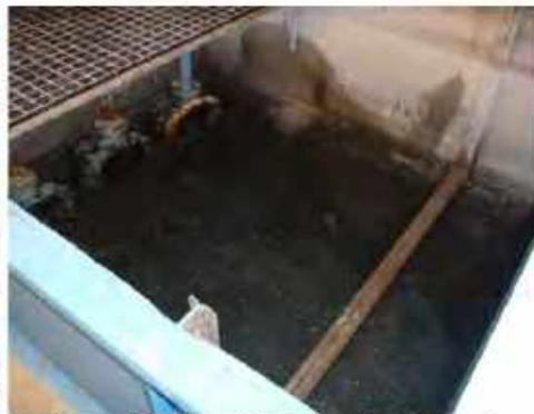
Image 66: Surge Tank During Normal Operation
