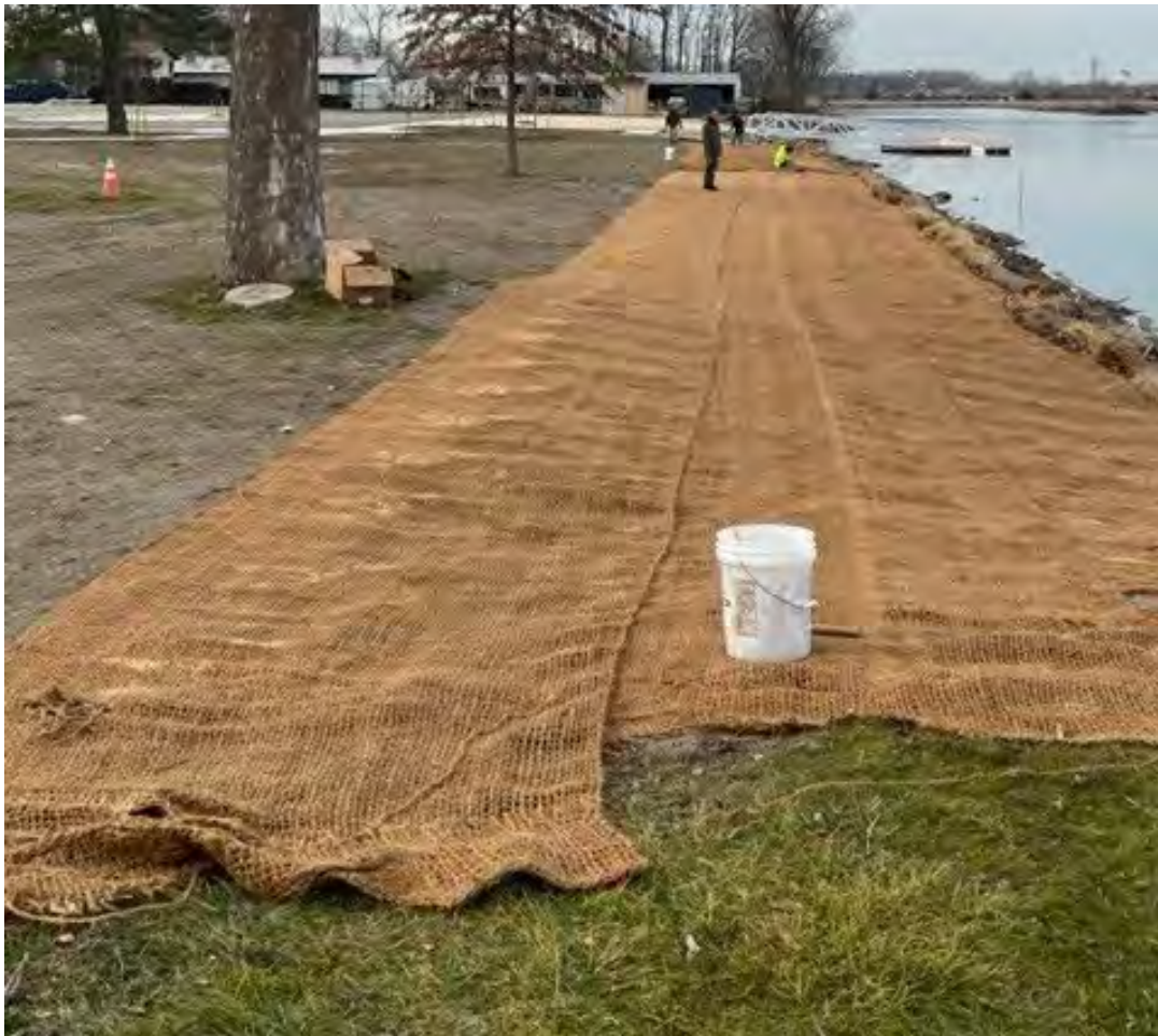
Figure 4: Shoreline erosion protection at Lake St. Clair Metropark, as part of the US Forestry Service and Great Lakes Restoration Initiative (GLRI) grant project to enhance the filtration of runoff waters into the Black Creek Marsh. 207/512
