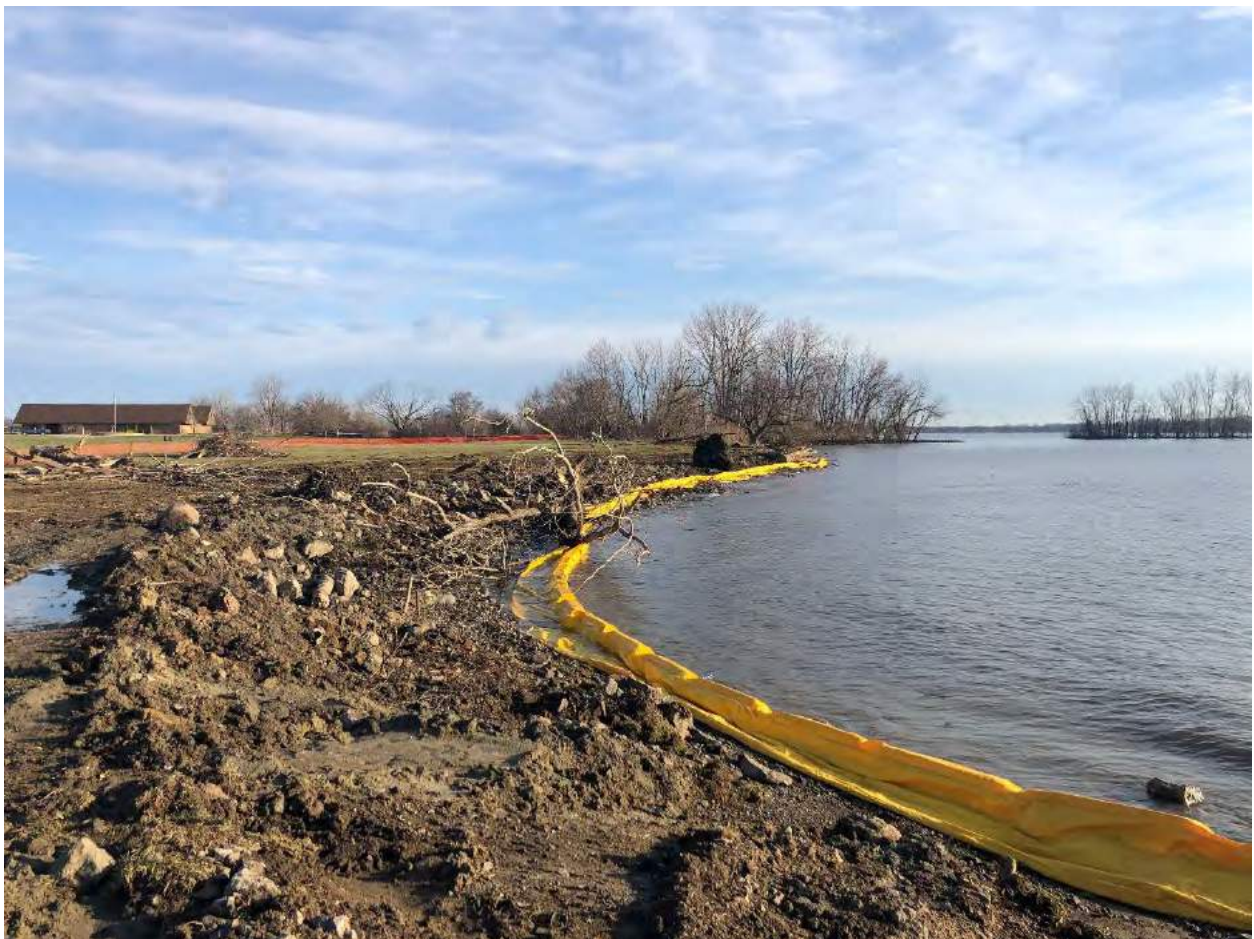
Figure 2: Shoreline restoration project at Lake Erie Metropark has begun. The shoreline has been graded to soften the slope, concrete rip rap has been removed, and woody debris has been incorporated.
