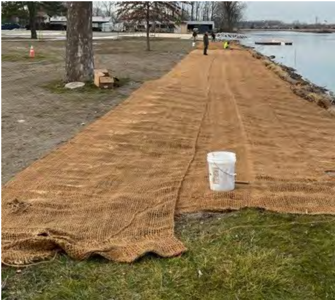
Figure 4: Shoreline erosion protection at Lake St. Clair Metropark, as part of the US Forestry Service and Great Lakes Restoration Initiative (GLRI) grant project to enhance the filtration of runoff waters into the Black Creek Marsh. 207/512
