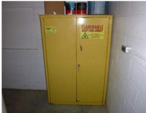
Image 71: Chemical Storage Closet
