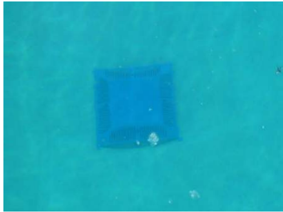
Pool drain not flush to pool surface
