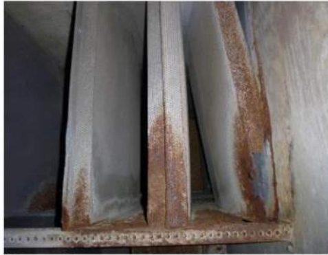
Image 82: Corroded Baffles in Equipment Room
