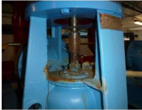
Image 58: Corrosion at Vertical In-Line Split Coupled Pump
