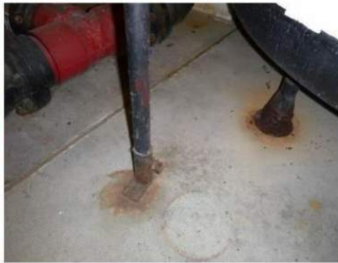
Image 50: Corrosion at Filter Support Leg
