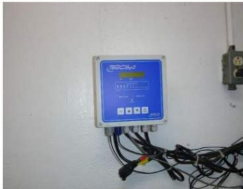
Image 75: Water Chemistry Controller
