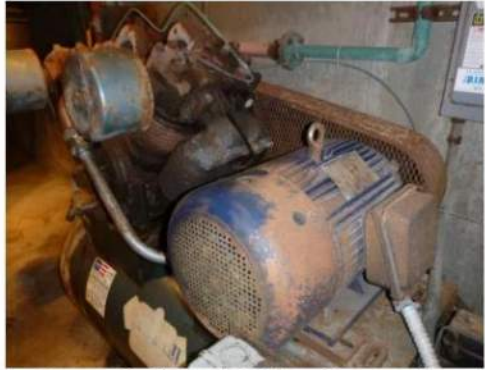
Image 80: Corroded Wave System Air Compressor
