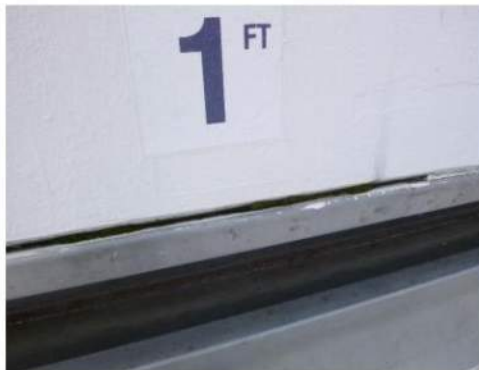
Image 16: Deterioration of Sealant Above Gutter and Concrete
