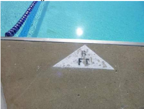
Damaged depth marker
