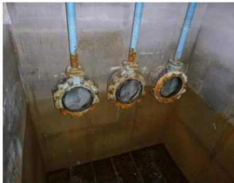
Image 37: Surge Tank Valves
