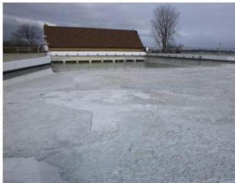
Image 1: Wave Pool Deteriorated Finish & Substrate
