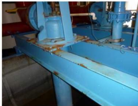
Image 64: Corrosion at Coated Steel Surge Tank
