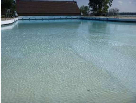
Visible repairs to the pool surface
