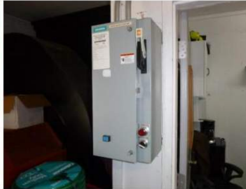
Image 62: Sprayground Pump Starter
