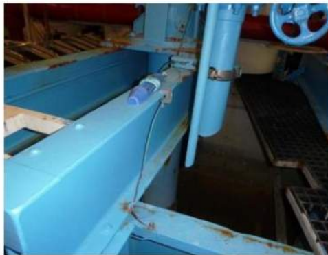
Image 65: Make-up Water Fill at Surge Tank
