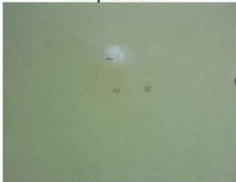
Image 7: Finish Discoloration & Degradation
