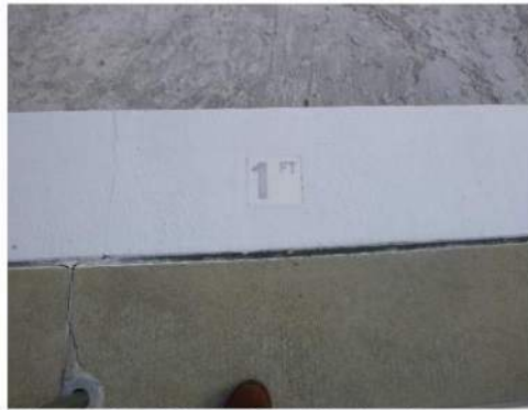
Image 35: Missing Deck Sealant between Pool Wall and Deck
