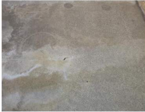
Image 32: Deck Discoloration Likely from Standing Water
