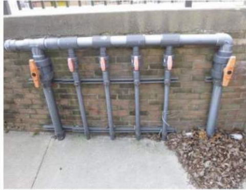
Image 46: Sprayground Feature Manifold
