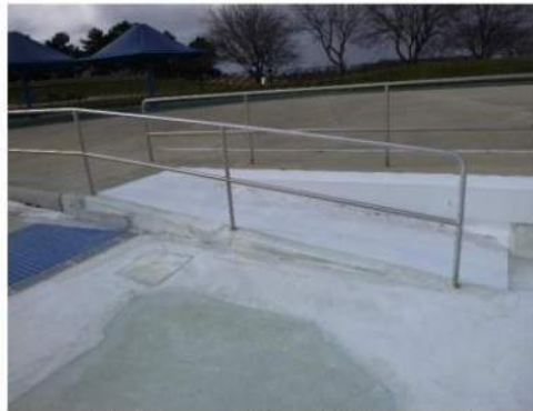
Image 21: Noncompliant ADA Ramp Entry
