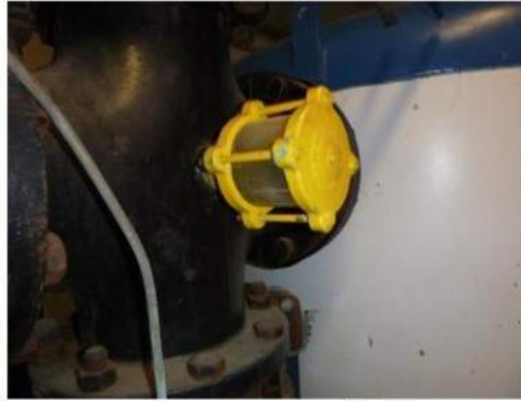
Image 54: Backwashing Sight Glass
