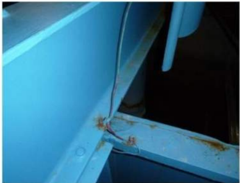
Image 59: Wave Pool System Bond Wiring
