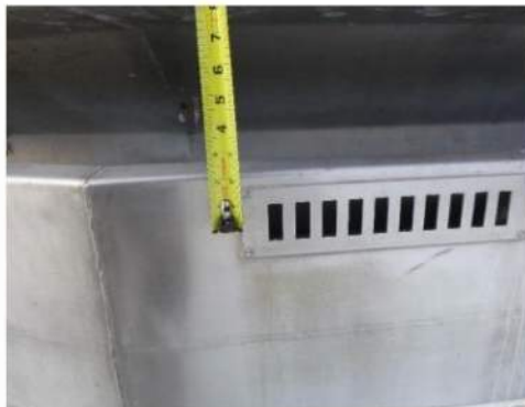
Image 15: Surge Weir and Gutter Hand Hold
