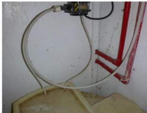
Image 74: Acid Feed Pump and Poly Piping
