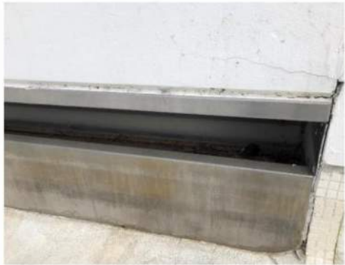
Image 13: Discoloration on Face of Stainless Steel Gutter Trough
