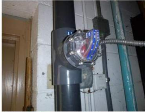
Image 45: Sprayground Flo-Vis Flow Meter
