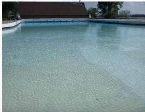
Image 8: Finish Condition in Submerged and Operating Condition
