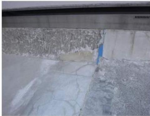
Image 5: Finish & Substrate Deterioration at Expansion Joint
