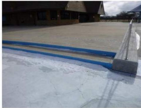
Image 6: Hairline Surface Cracking at Step Entry
