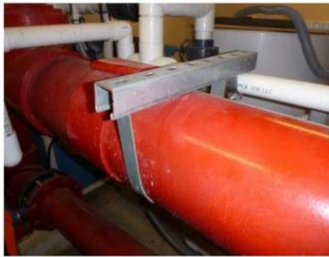
Image 47: Unsupported Strut and Pipe Guides / Straps
