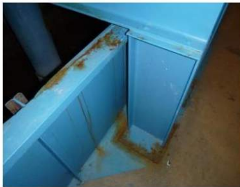
Image 63: Corrosion at Coated Steel Surge Tank
