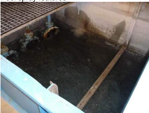
Wave pool surge pit
