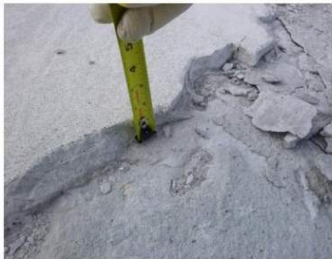
Image 3: Delaminated Plaster Finish
