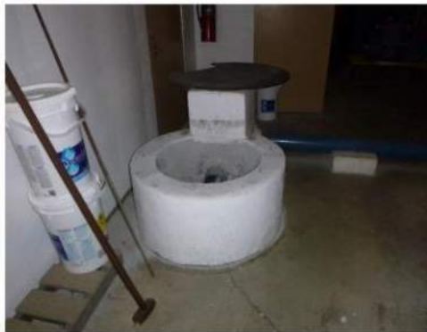
Image 52: Sanitary Waste Pit
