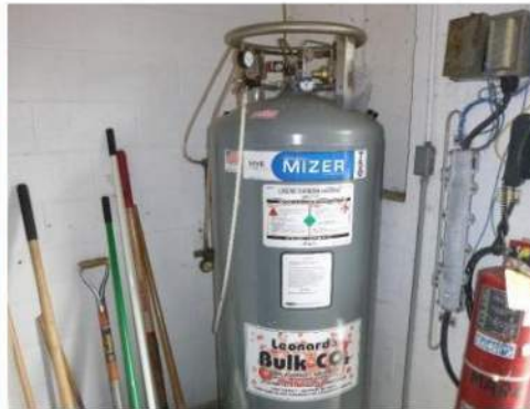
Image 68: Bulk Carbon Dioxide Tank
