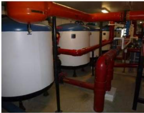
Image 49: Vertical Sand Filtration Tanks
