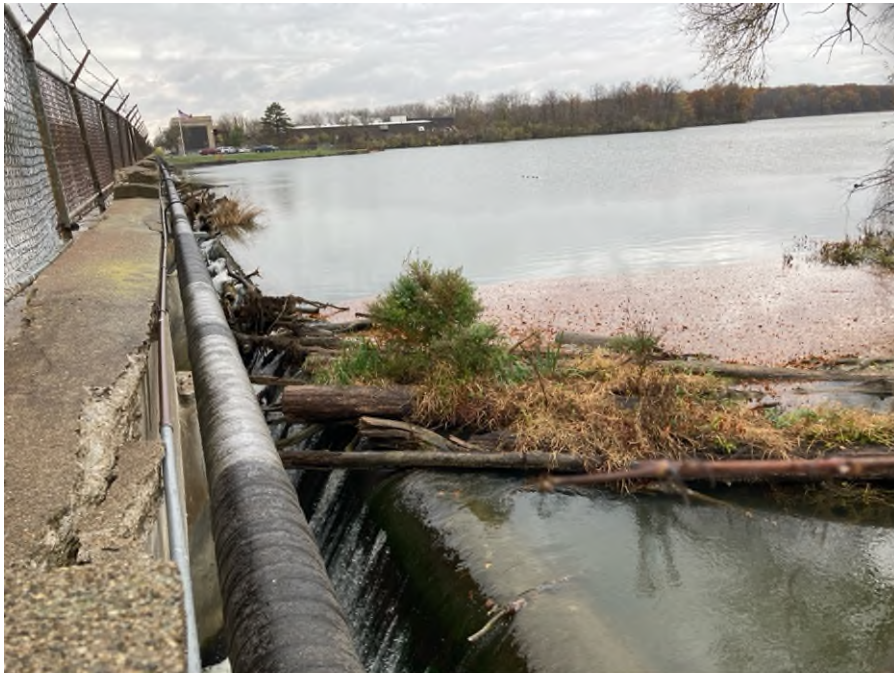
Photo #3: Principal Spillway Weir Wall. Issue: Debris, Action: Maintenance.
