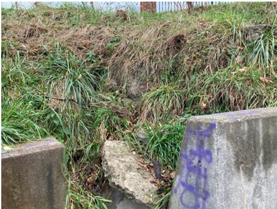
Photo #34: Embankment Downstream Slope. Right above storm sewer from Rhodes. likely from seepage observed. Issue: Depression, Action: Maintenance.
