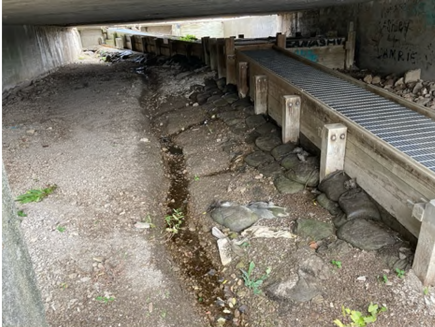
Photo #27: Fish Ladder Chute. Issue: Seepage, Action: Monitor. Type: Flow.
