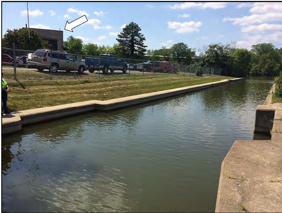
Photograph 6 – Earthen needle section located between lock and powerhouse Note the arrow indicating the location of the former powerhouse
