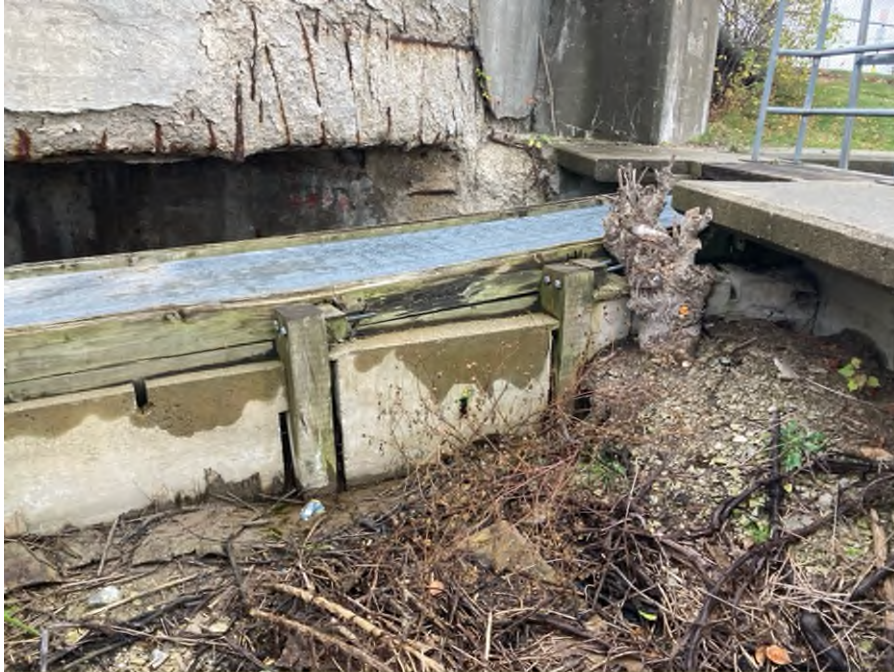
Photo #29: Fish Ladder Chute.
