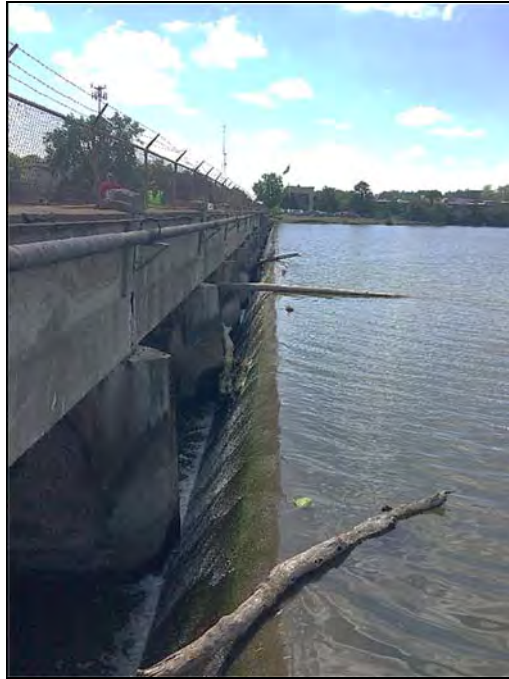
Photograph 7 – Principal spillway crest viewed from left Note the minor buildup of woody debris
