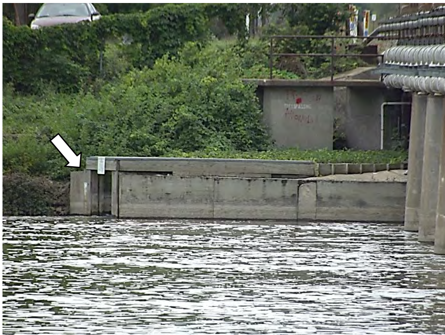
Photograph 8 – Downstream right principal spillway abutment wall. Note the outlet of the fish ladder.
