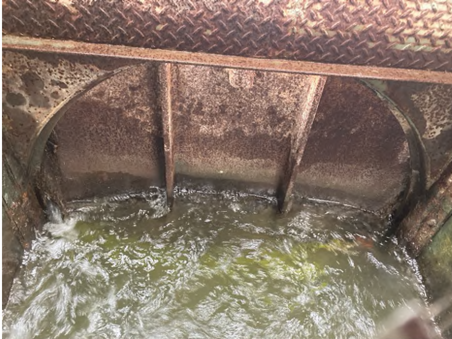
Photo #19: Fish Ladder Inlet Gate.
