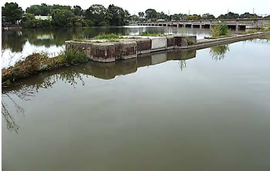
Photograph 12 – Upstream portion of lock wall viewed from right. Note the deteriorated concrete vegetation growing from cracks.
