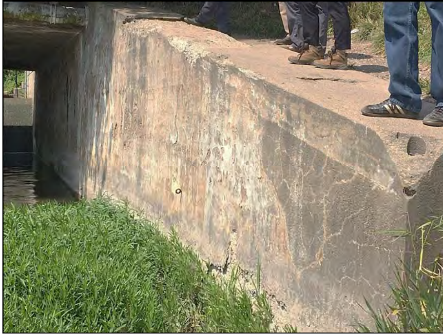
Photograph 9 – Downstream left spillway abutment wall Note the minor spalling and cracking
