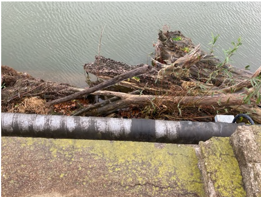
Photo #4: Principal Spillway Weir Wall. Issue: Debris, Action: Maintenance.
