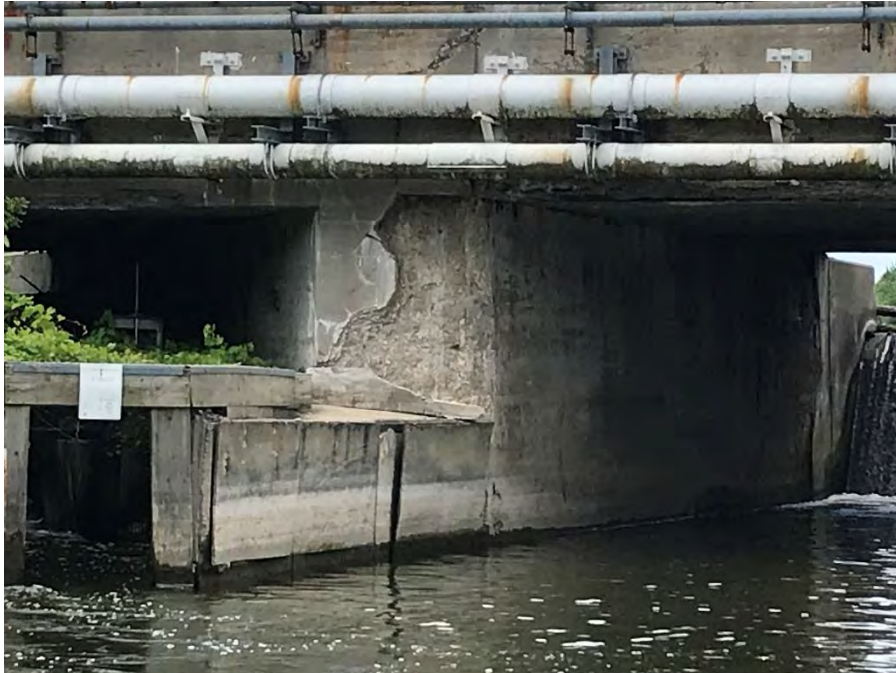
Photograph 11 – Right downstream abutment wall Note the spalling and delamination
