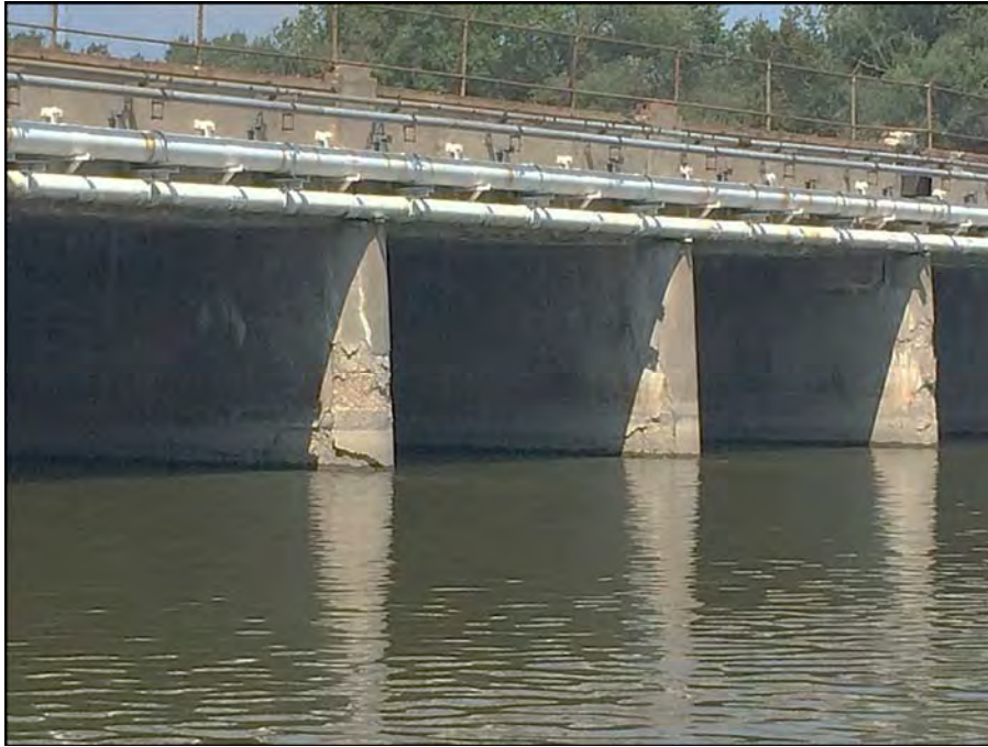
Photograph 13 – Typical spalling of bridge piers
