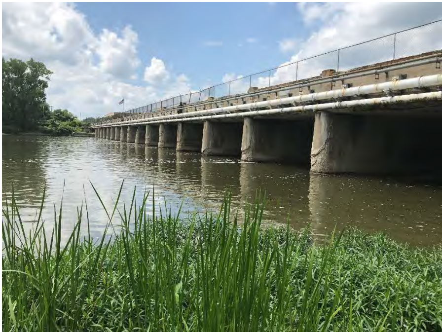
Photograph 14 – Downstream face of bridge over spillway Note the spalling and delamination of piers
