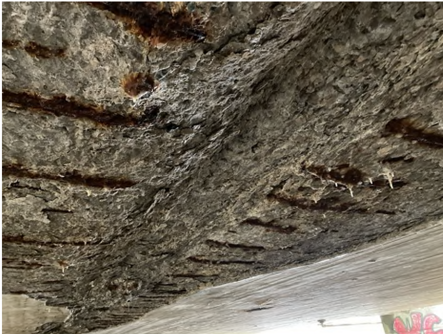
Photo #12: Principal Spillway Bridge. Issue: Deteriorating Material, Action: Maintenance. Material: Concrete.
