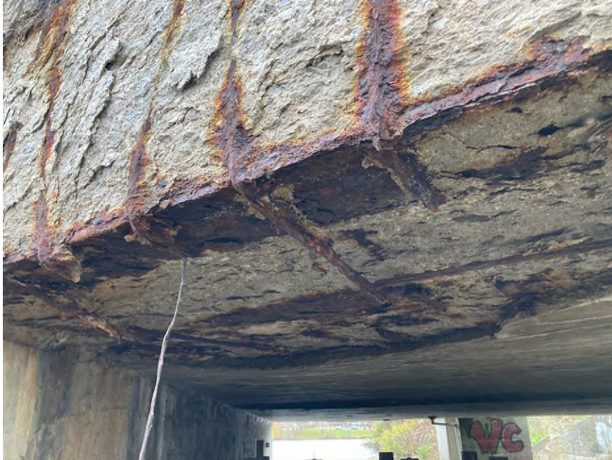
Photo #11: Principal Spillway Bridge. Issue: Deteriorating Material, Action: Maintenance. Material: Concrete.
