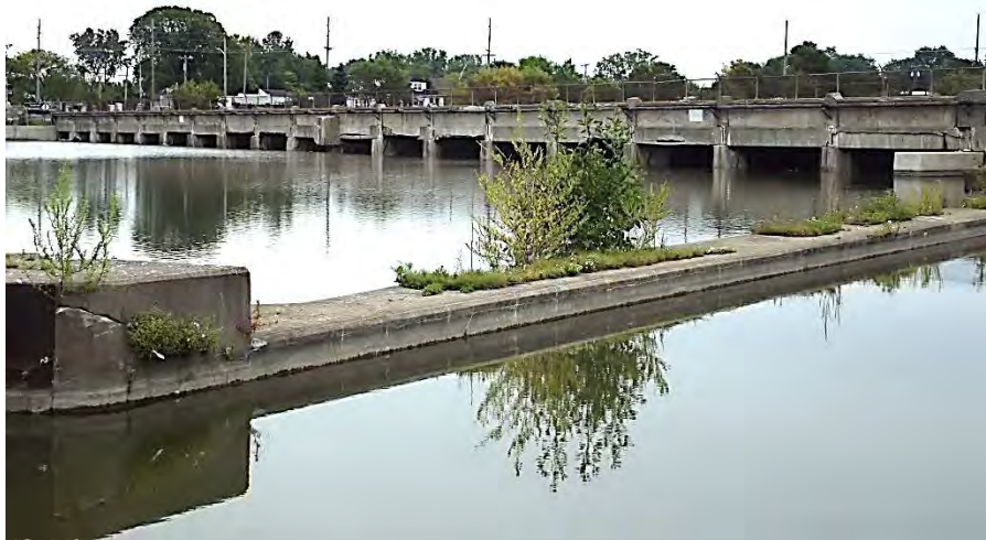
Photograph 13 – Downstream portion of lock wall viewed from right. Note the deteriorated concrete and vegetation growing from cracks.
