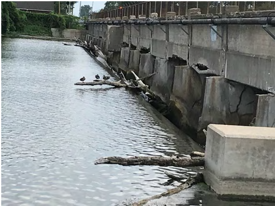
Photograph 8 – Spillway crest viewed from right Note the minor debris build up and delamination of bridge beams
