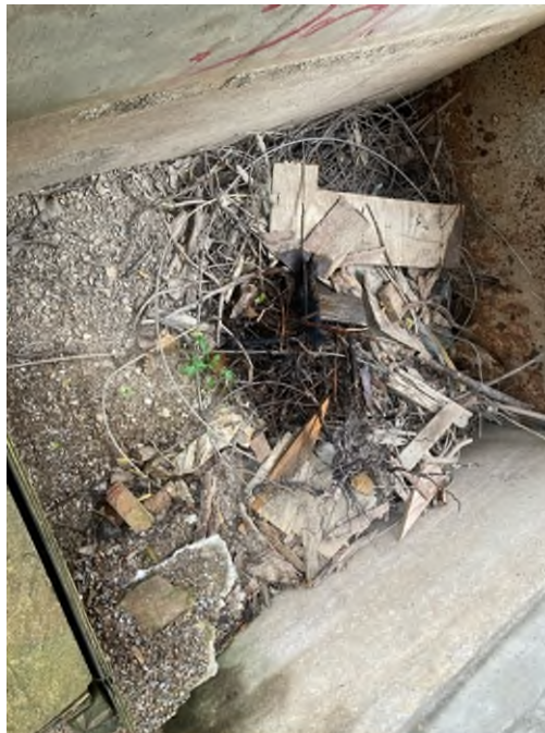
Photo #16: Fish Ladder Abandoned Conduit. Issue: Depression, Action: Maintenance.
