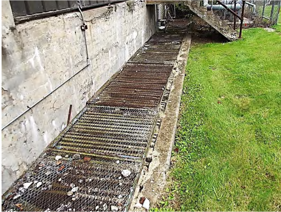
Photograph 19 – Channel along right powerhouse wall. Note that there was flow through this channel on the date of the inspection.
