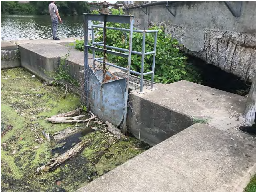
Photograph 18 – Right lock gate and operator Note that this gate acts as the inlet to the DNR fish ladder
