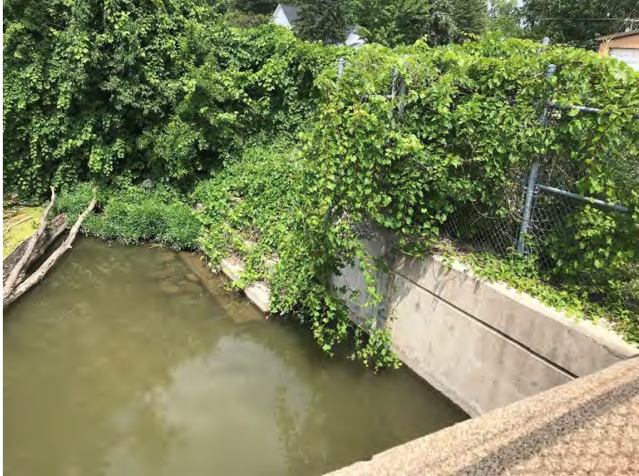
Photograph 10 – Left upstream abutment wall Note the overgrowth of vegetation
