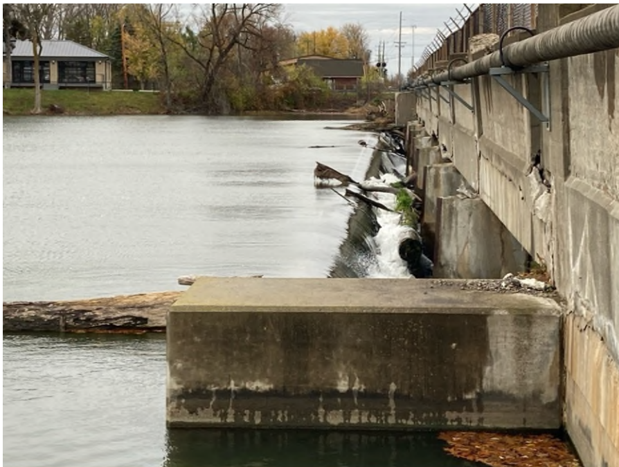
Photo #6: Principal Spillway Weir Wall. Issue: Debris, Action: Maintenance.
