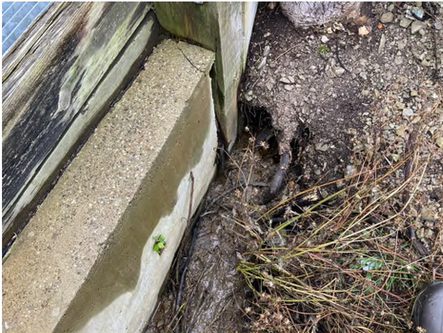
Photo #28: Fish Ladder Chute. Issue: Seepage, Action: Monitor. Type: Flow.
