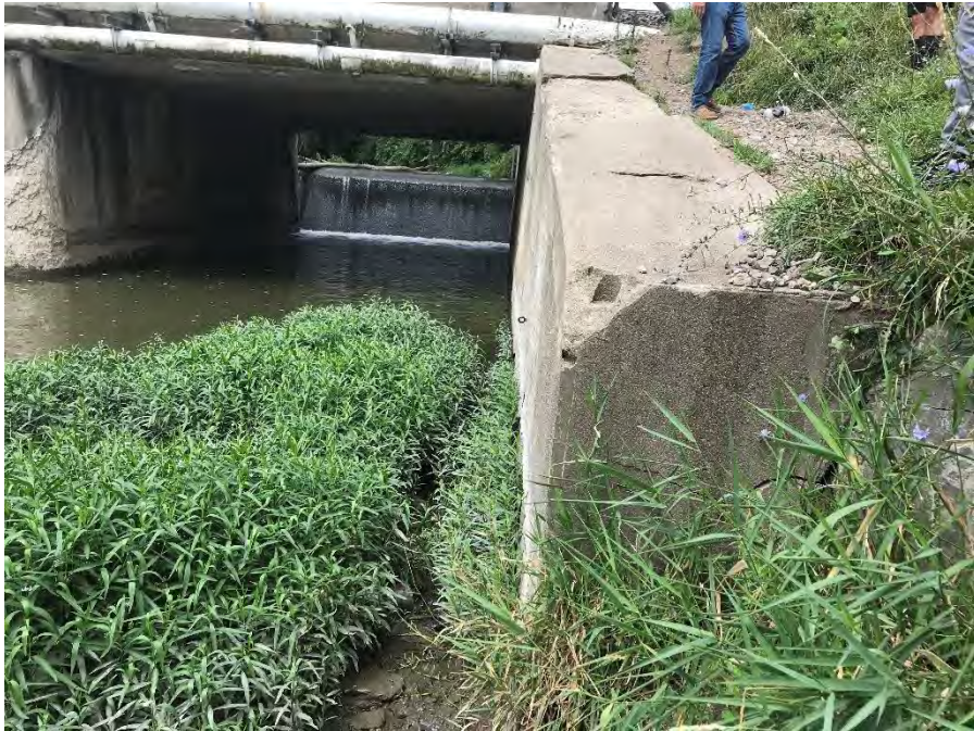
Photograph 12 – Left downstream abutment wall Note the spalling
