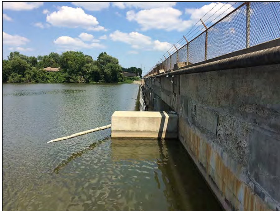
Photograph 10 – Upstream right spillway abutment wall Note that a portion of this wall was recently reconstructed
