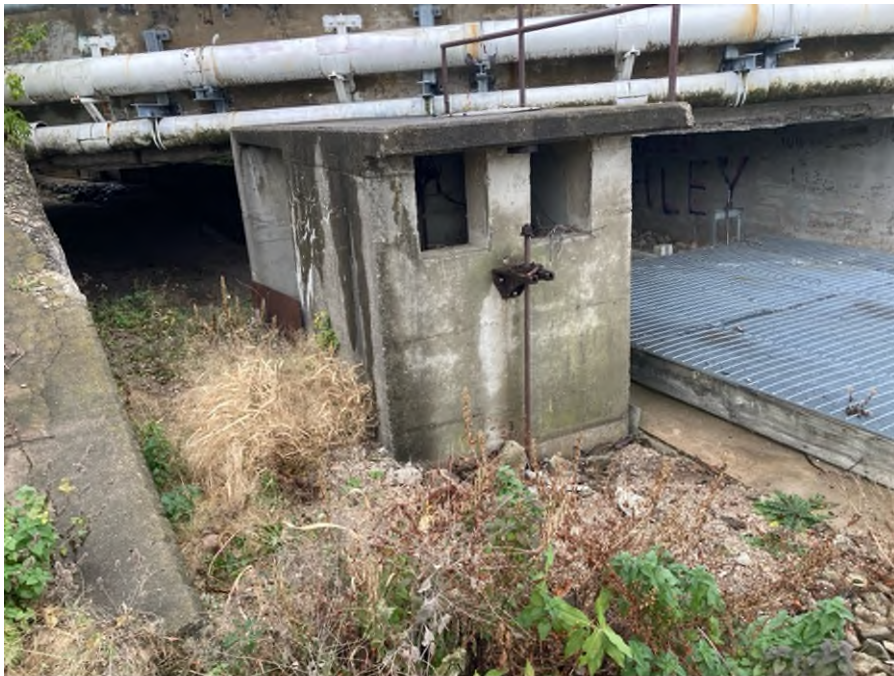
Photo #24: Fish Ladder Abandoned Gate.
