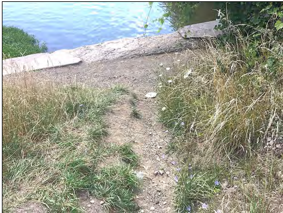
Photograph 6 – Downstream face of left abutment viewed from left Note the foot traffic erosion
