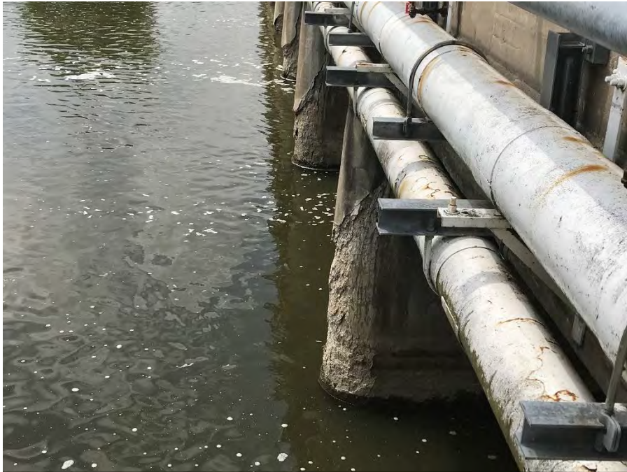
Photograph 15 – Typical pier spalling and delamination
