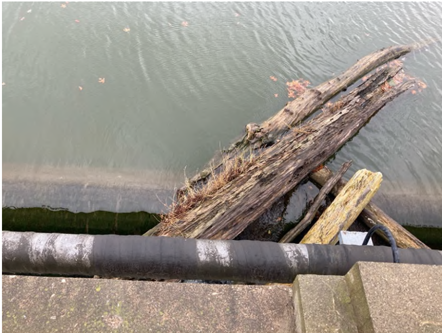
Photo #5: Principal Spillway Weir Wall. Issue: Debris, Action: Maintenance.
