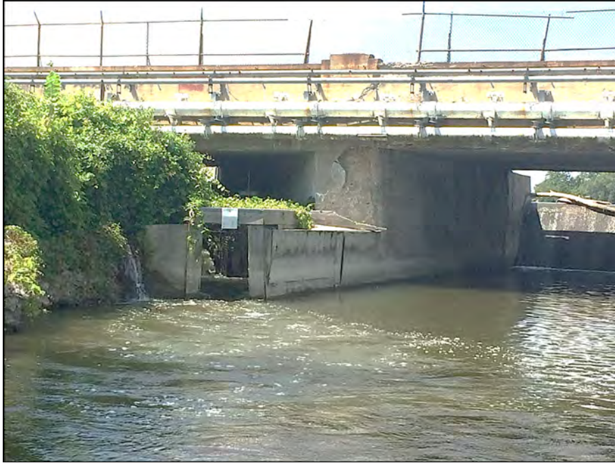
Photograph 11 – Downstream right spillway abutment wall Note the spalling and fish ladder outlet
