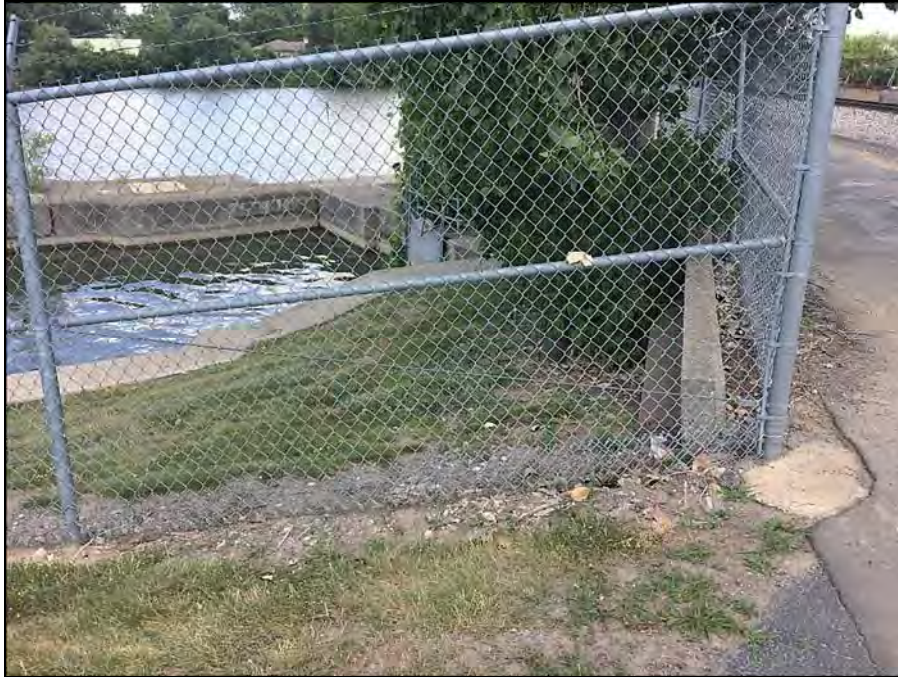
Photograph 1 – Upstream face of right abutment viewed from right Note the small trees and brush near the spillway structure
