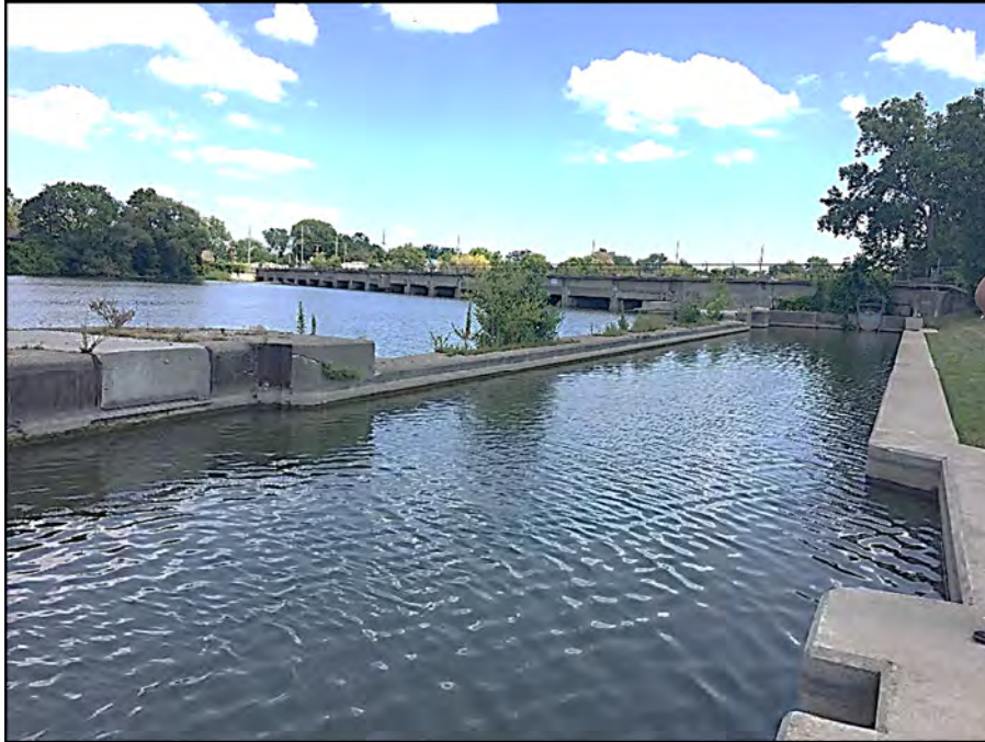
Photograph 15 – Abandoned lock viewed from upstream Note that the right wall was recently reconstructed
