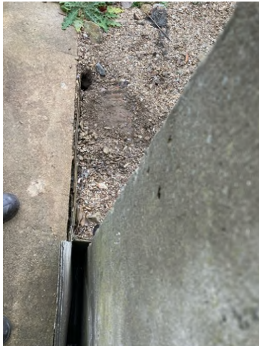
Photo #17: Fish Ladder Abandoned Conduit. Issue: Sink Hole, Action: Maintenance.
