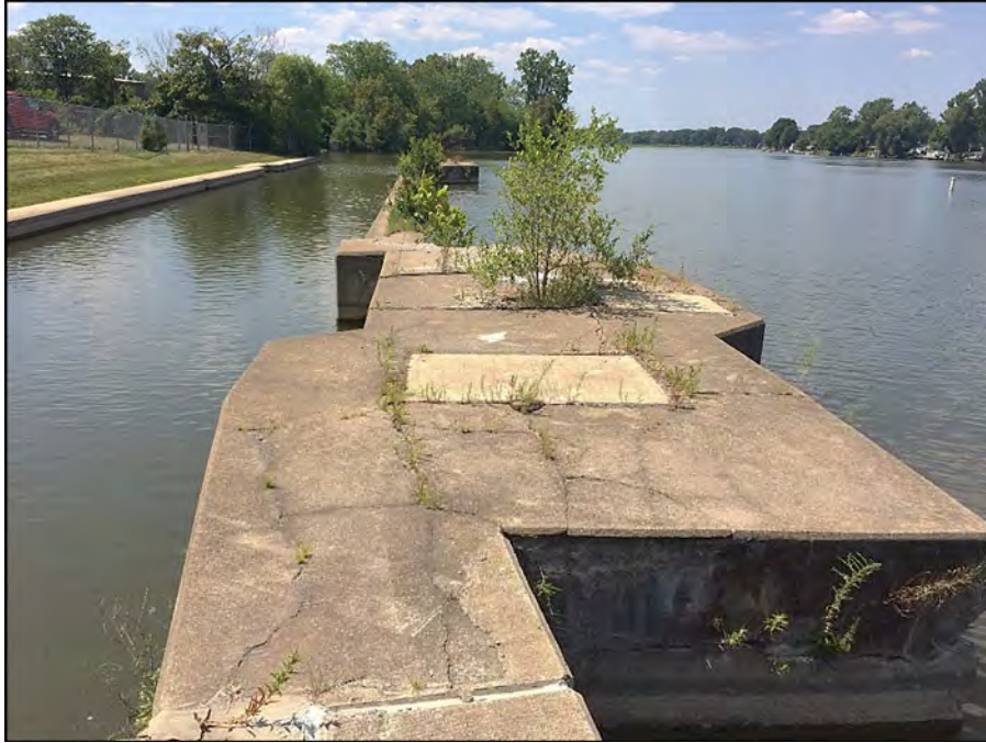
Photograph 17 – Left wall of abandoned lock Note that this is the original wall and shows signs of deterioration
