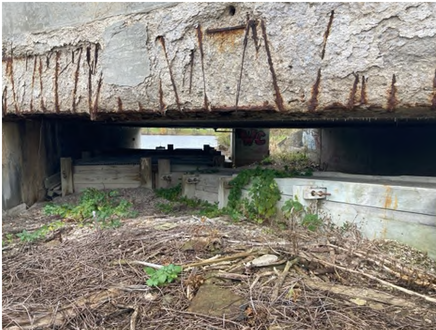
Photo #30: Fish Ladder Chute.
