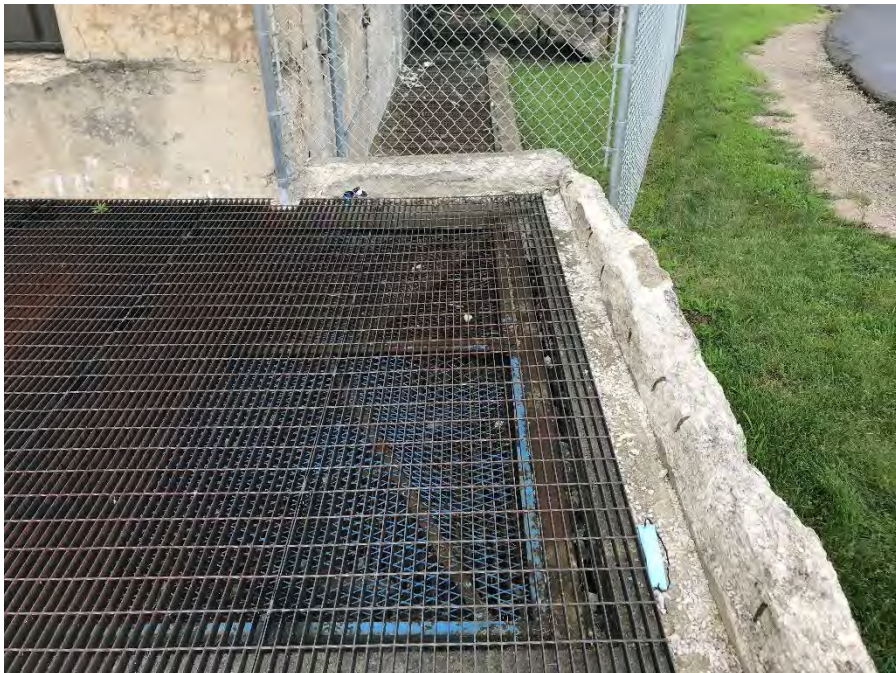
Photograph 24 – Bypass channel at left of powerhouse Note that there was flow through this channel during this inspection
