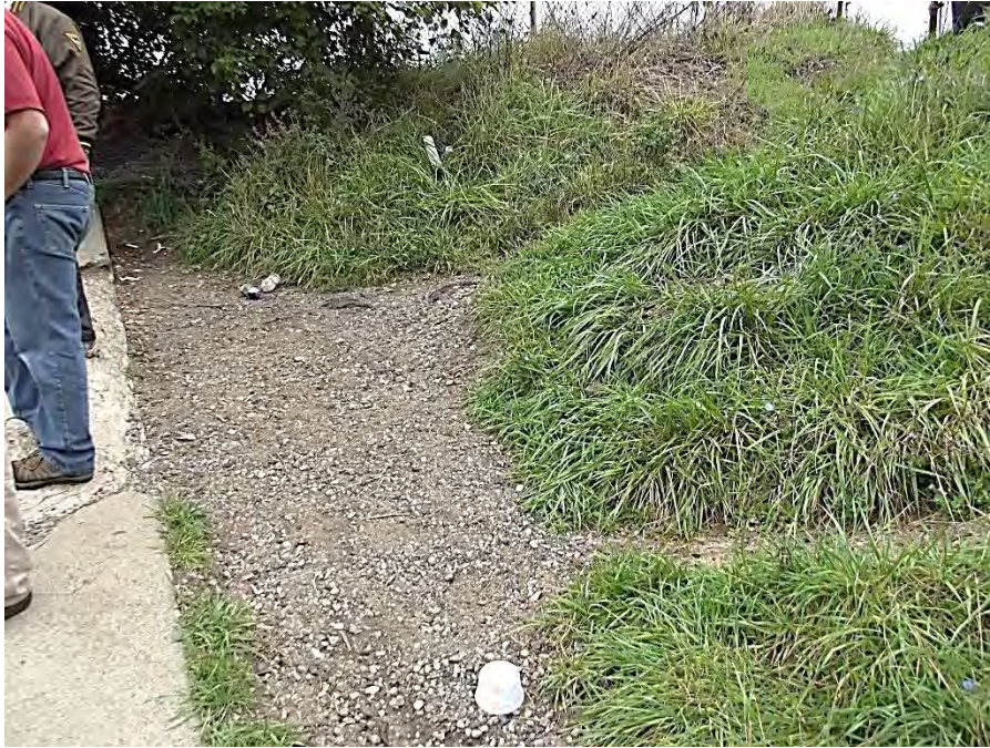
Photograph 5 – Downstream face of left embankment viewed from left. Note the foot traffic erosion.
