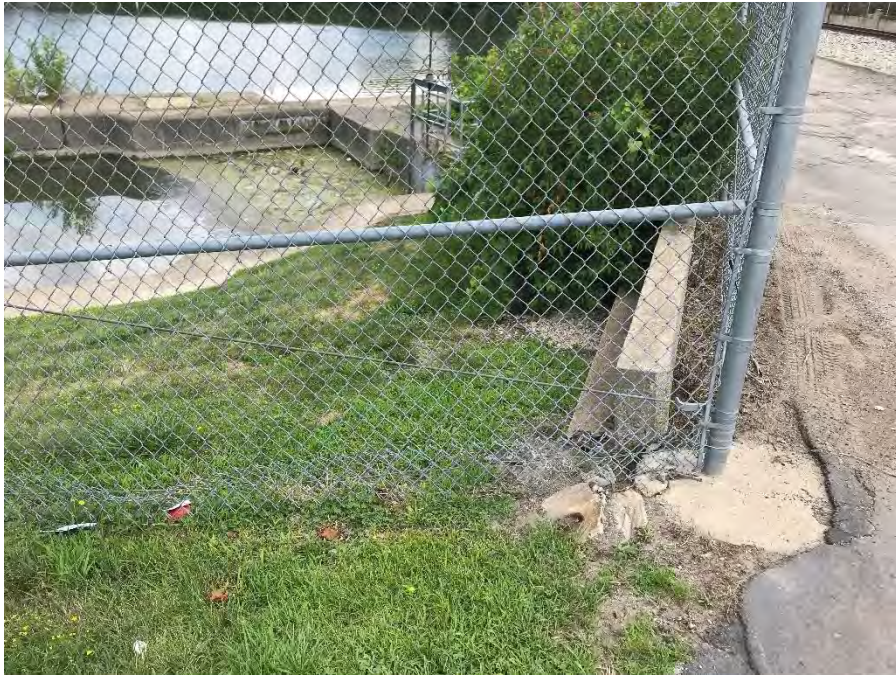
Photograph 1 – Upstream face of right abutment viewed from right Note the brush growth
