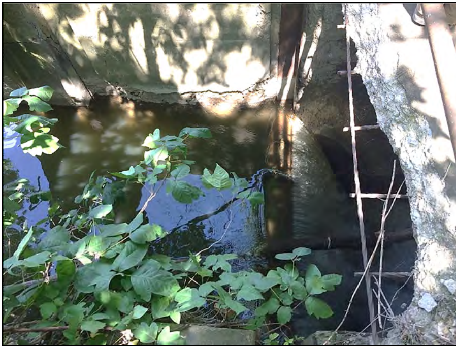
Photograph 20 – Small powerhouse head gate viewed from right Note the deteriorated concrete and exposed reinforcing steel
