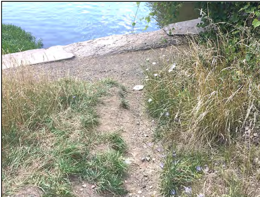
Photograph 4 – Left abutment viewed from left Note the foot traffic erosion
