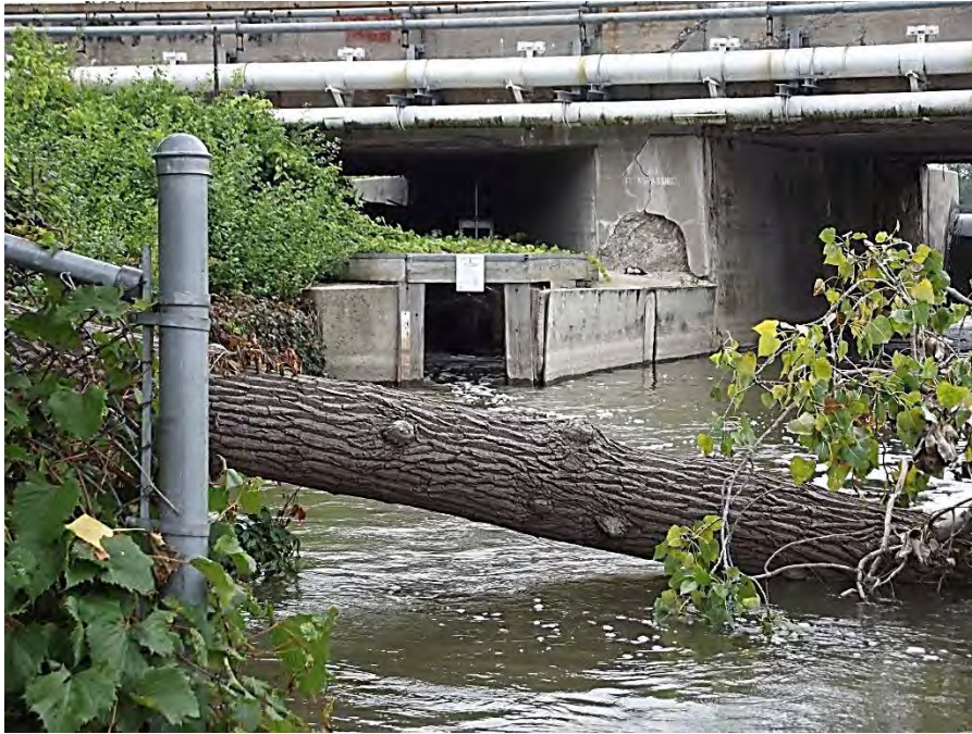
Photograph 17 – Fish ladder outlet viewed from downstream. Note the overgrowth of vegetation.
