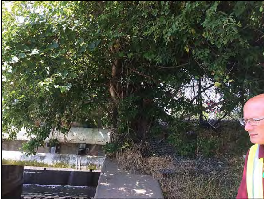
Photograph 5 – Trees growing from left abutment
