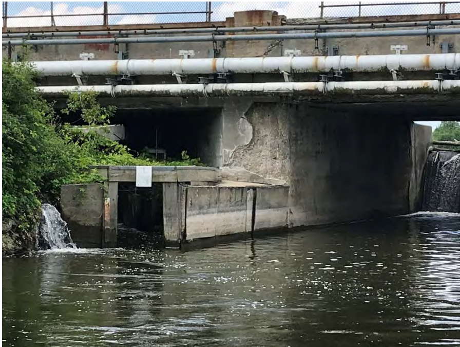
Photograph 21 – DNR fish ladder outlet Note the major leaking at right wall
