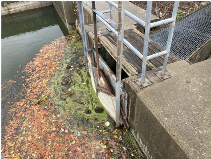
Photo #18: Fish Ladder Inlet Gate.
