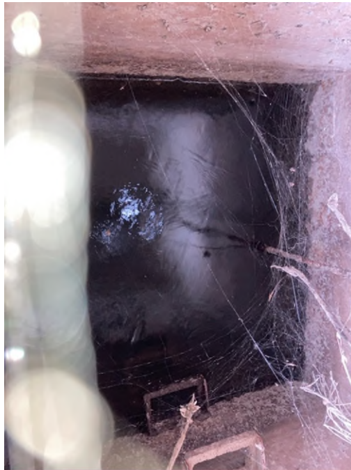
Photo #25: Fish Ladder Abandoned Gate Flow observed through gate.
