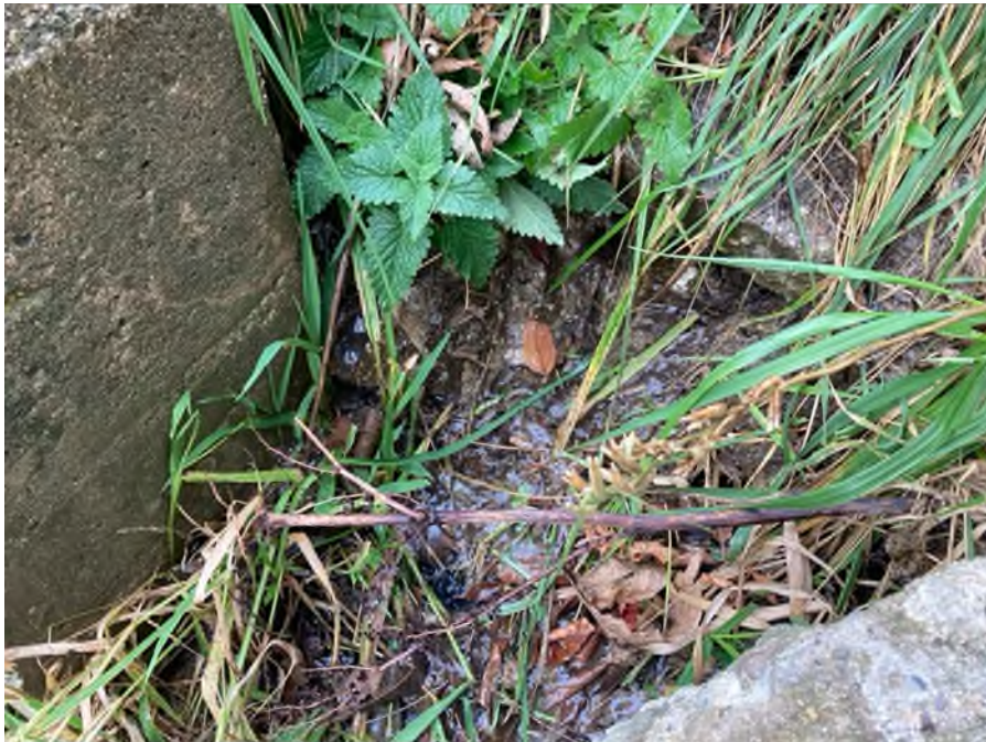
Photo #33: Embankment Downstream Slope. Might be from storm sewer. Issue: Seepage, Action: Monitor. Type: Flow.
