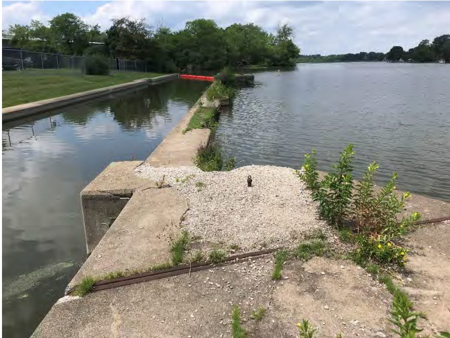
Photograph 17 – Left abutment wall of abandoned lock Note the spalling and cracking
