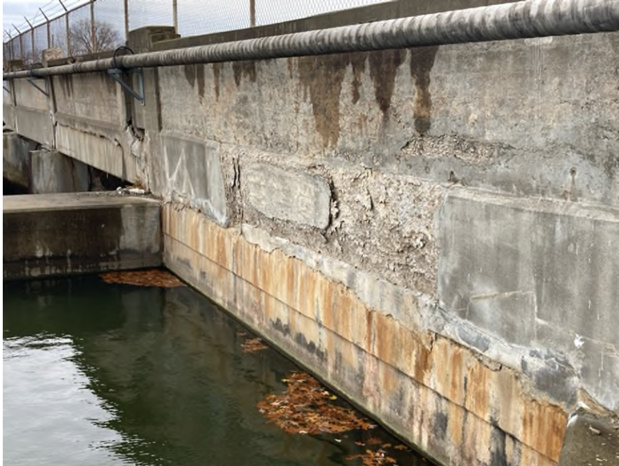
Photo #9: Principal Spillway Abutment Right Wall. Issue: Deteriorating Material, Action: Maintenance. Material: Concrete.
