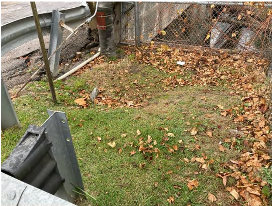
Photo #32: Embankment Upstream Slope. Issue: Depression, Action: Maintenance.
