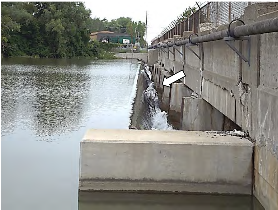
Photograph 6 – Principal spillway crest viewed from right. Note the minor debris build up.
