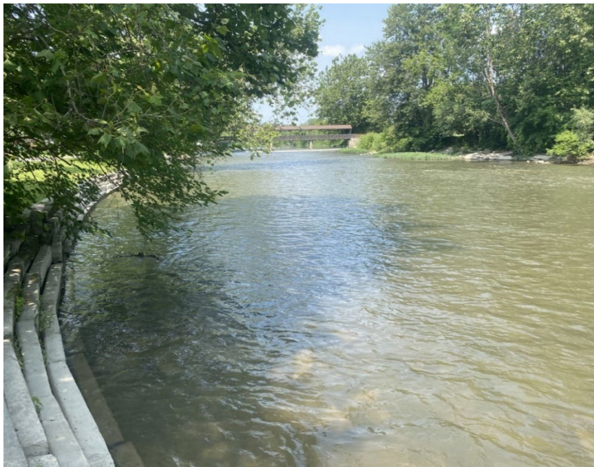
Photograph 2: View north of concrete walls/steps extending to the edge of the Huron River downstream of the Flat Rock Dam.
