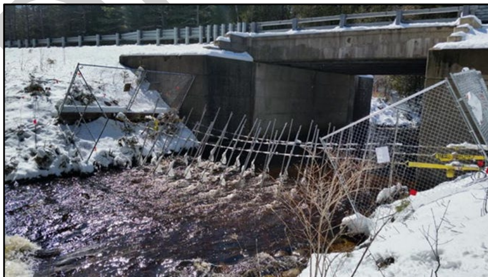
Figure 20: Electrical Barrier (Johnson et al., 2021)
